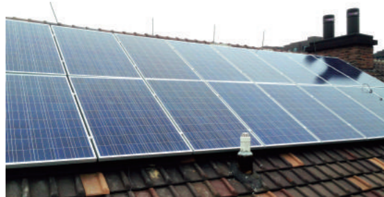
Hangzhou Hejiayuan Residential Solar System 6kW
