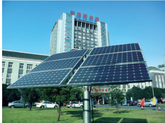
Hangzhou East Software Park Commercial Solar System 1.5kW
