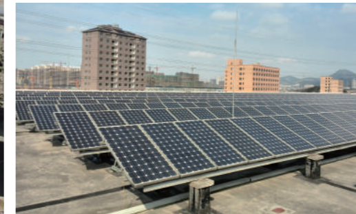
Shanghai Kangshun Industrial Solar Systems 1.2MW
