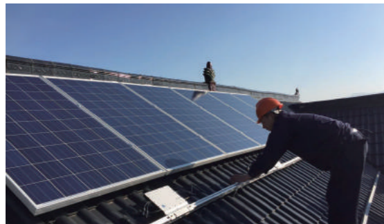
Quzhou Shiliang Residential Solar System 5kW
