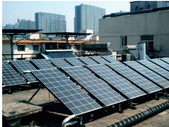
Hangzhou Energy Institute Commercial Solar System 10kW
