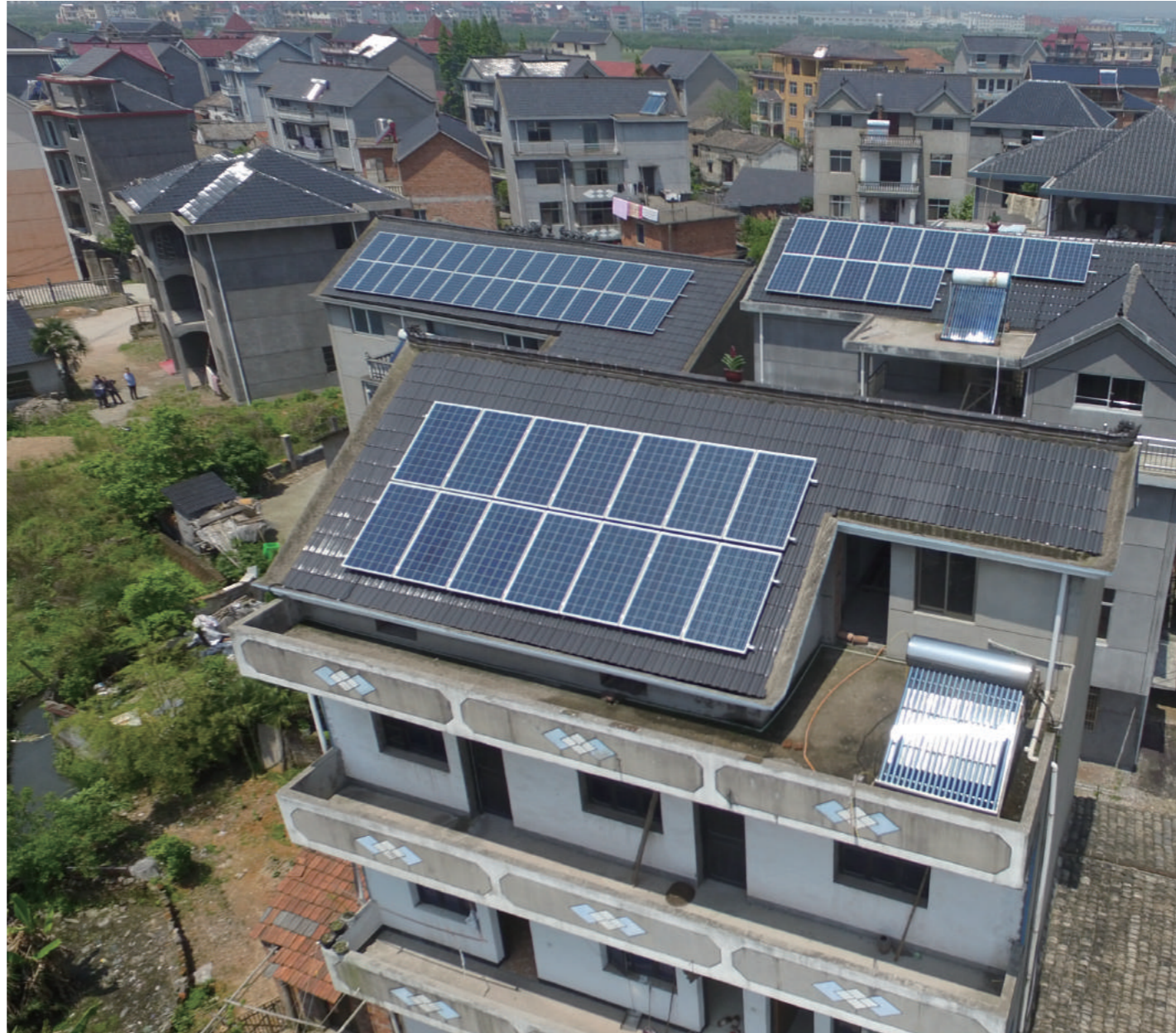
Quzhou Qujiang District Nieli Town 500 Residential Solar Systems 500 x 3kW
