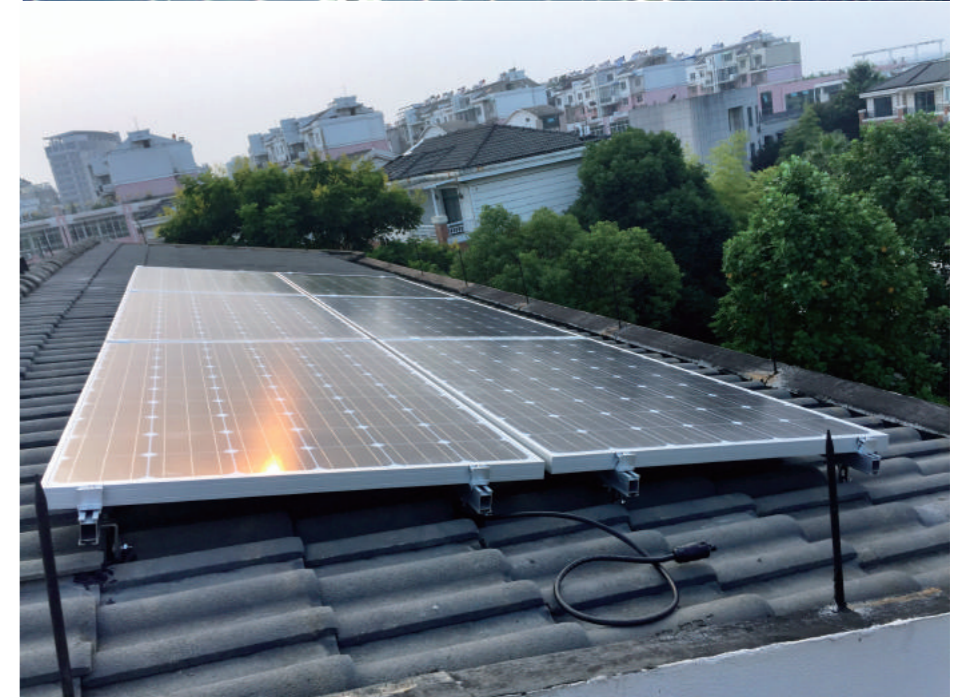
Quzhou Villa Residential Solar System 2kW
