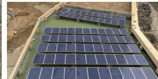
Hangzhou Xie' an Zijun Commercial Solar System 22kW
