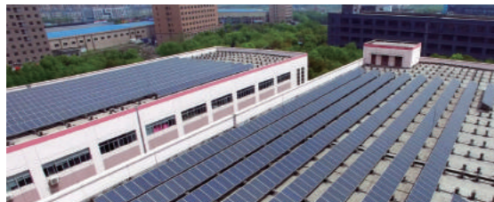
Hangkai Group Industrial Solar Systems 200kW
