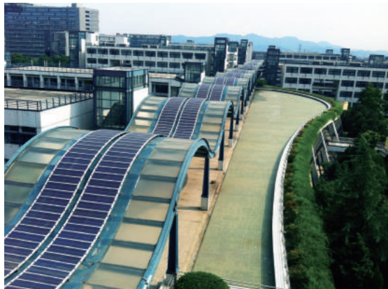
Zhejiang University Commercial Solar System 70kW
